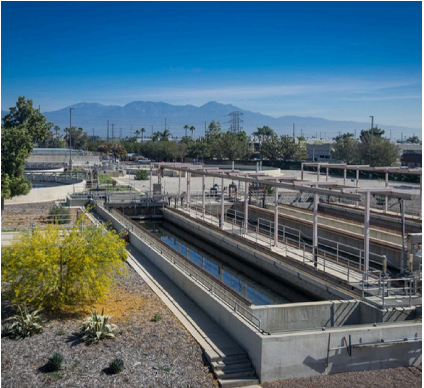
Carbon Canyon Water Recycling Facility (CCWRF) in Chino, CA - Water is filtered to remove suspended organic solids and is disinfected using sodium hypochlorite.
