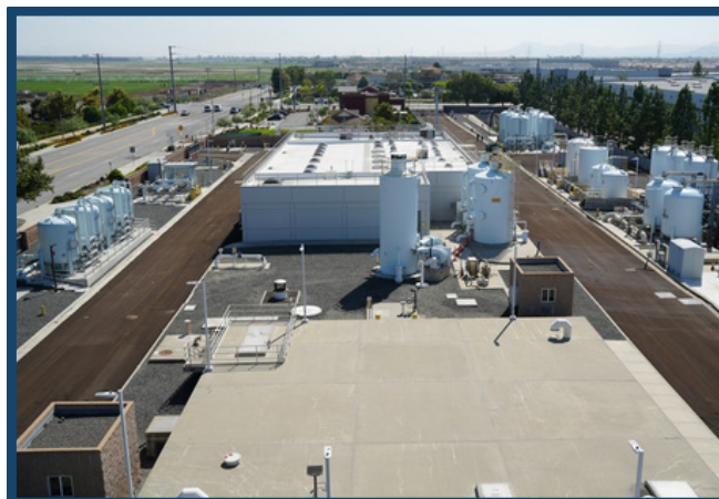
The Chino I Desalter processes up to 14 million gallons per day (MGD) of groundwater from the Chino Basin using reverse osmosis, ion exchange, air stripping, and granular activated carbon treatment processes.
