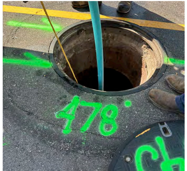
Task A (Photo A8): View of IEUA markings noting flow direction and distance of pipeline segment to alert field operators.
