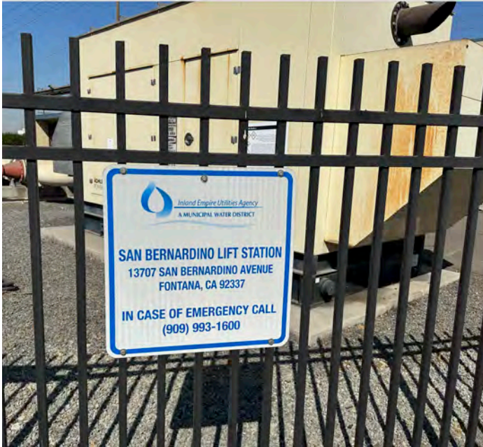
Task B (Photo B1): Inspection of San Bernardino Lift Station planned for complete capital upgrade in 2025-2026.
