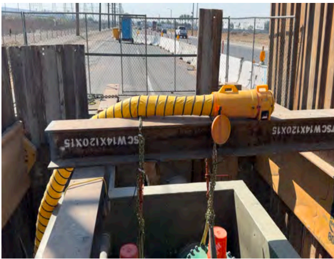
Task B (Photo C3): Inspection of Regional Force Main construction site manhole structure site (view 1).
