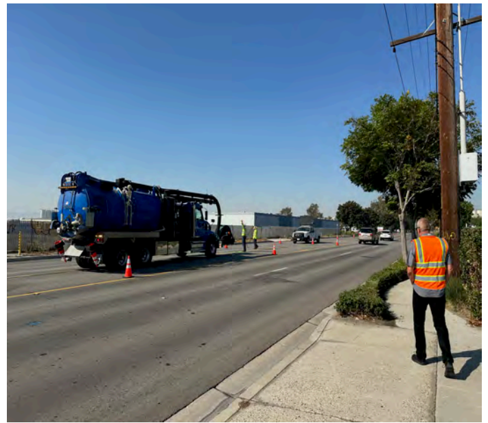
Task A (Photo A4): View of IEUA combination truck preparing for siphon cleaning operations facing west in roadway with traffic control measures in place.
