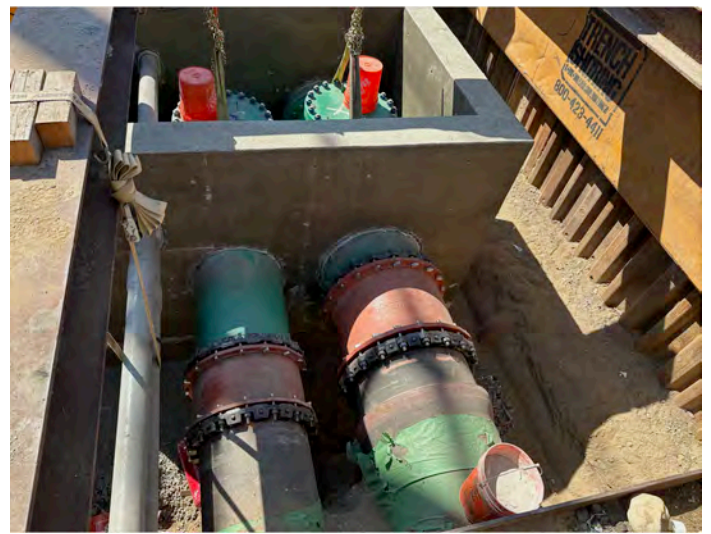
Task B (Photo C4): Inspection of Regional Force Main construction site manhole structure site (view 2).
