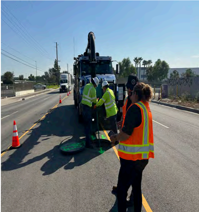
Task A (Photo A5): View looking east at Fontana Interceptor Siphon location during cleaning operations.
