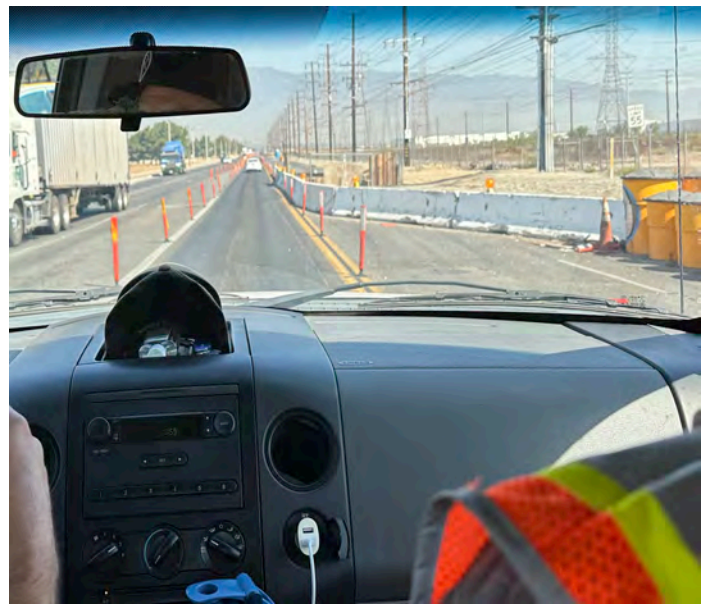
Task B (Photo C2): View of Regional Force Main construction site looking north.
