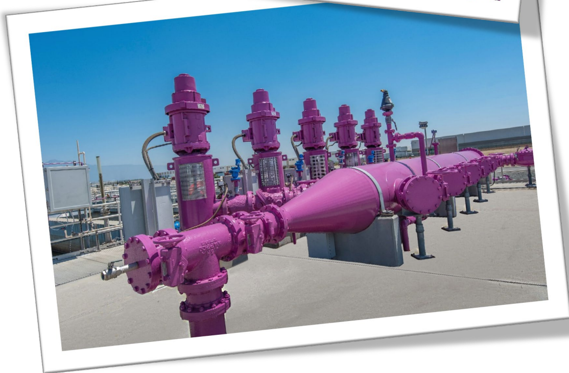
Regional Plant No. 5
