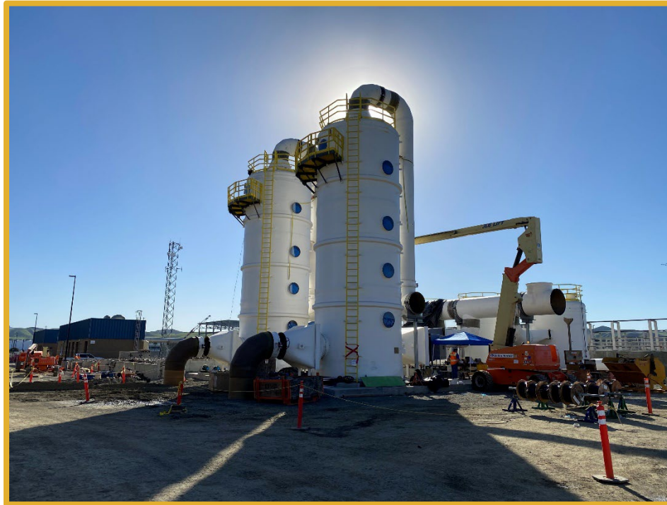
RP-5 Main Odor Control Facility
