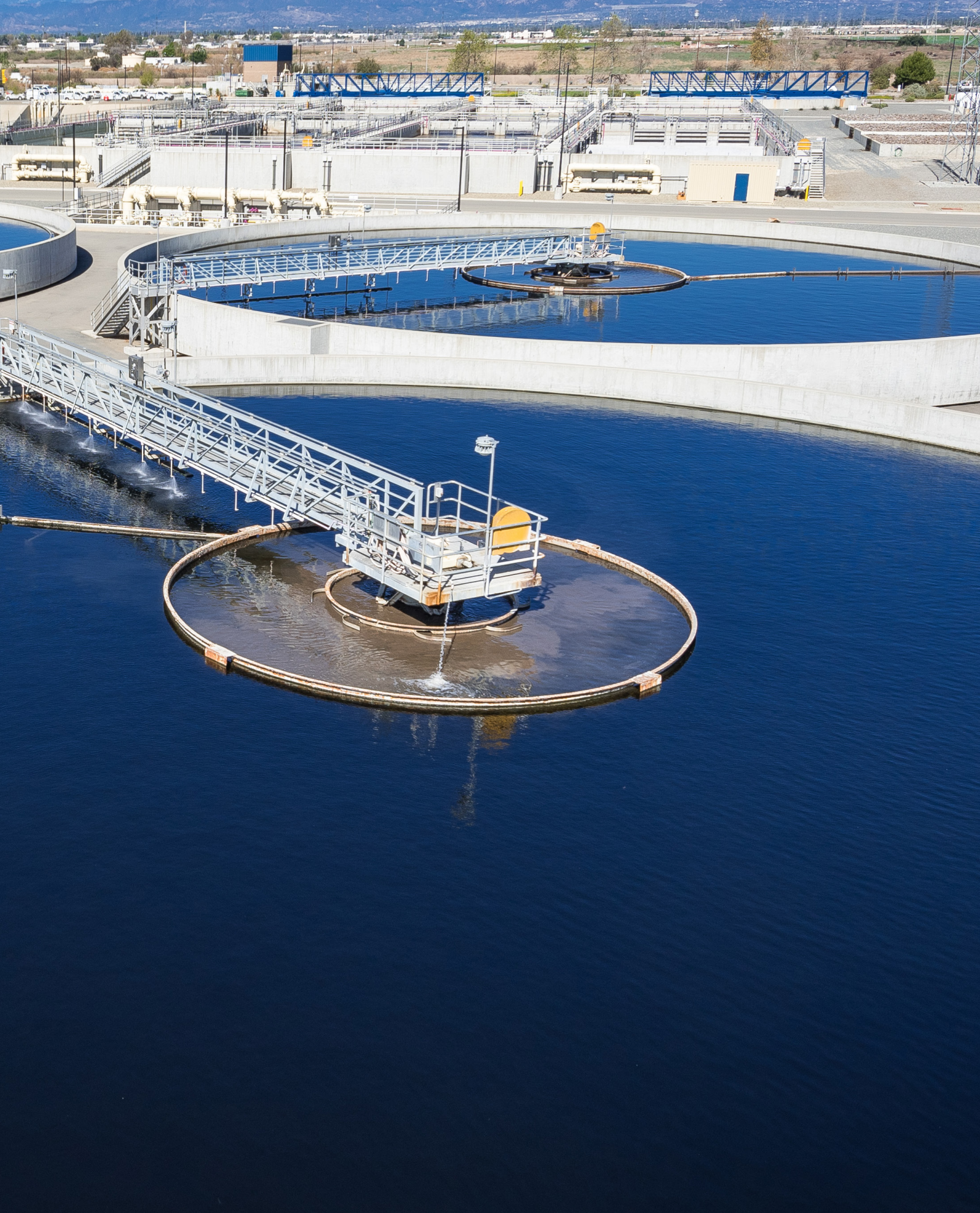
Regional Plant (RP)-5 in Chino, CA treats up to 15 million gallons of wastewater per day, equivalent to 22 Olympic-sized swimming pools.
