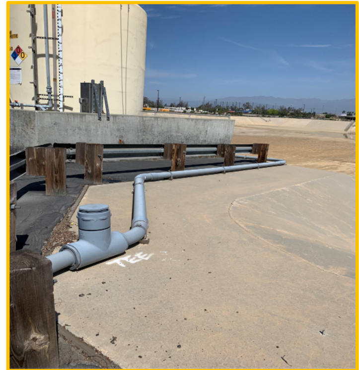
Temporary Sodium Hypochlorite (Bleach) Piping System
