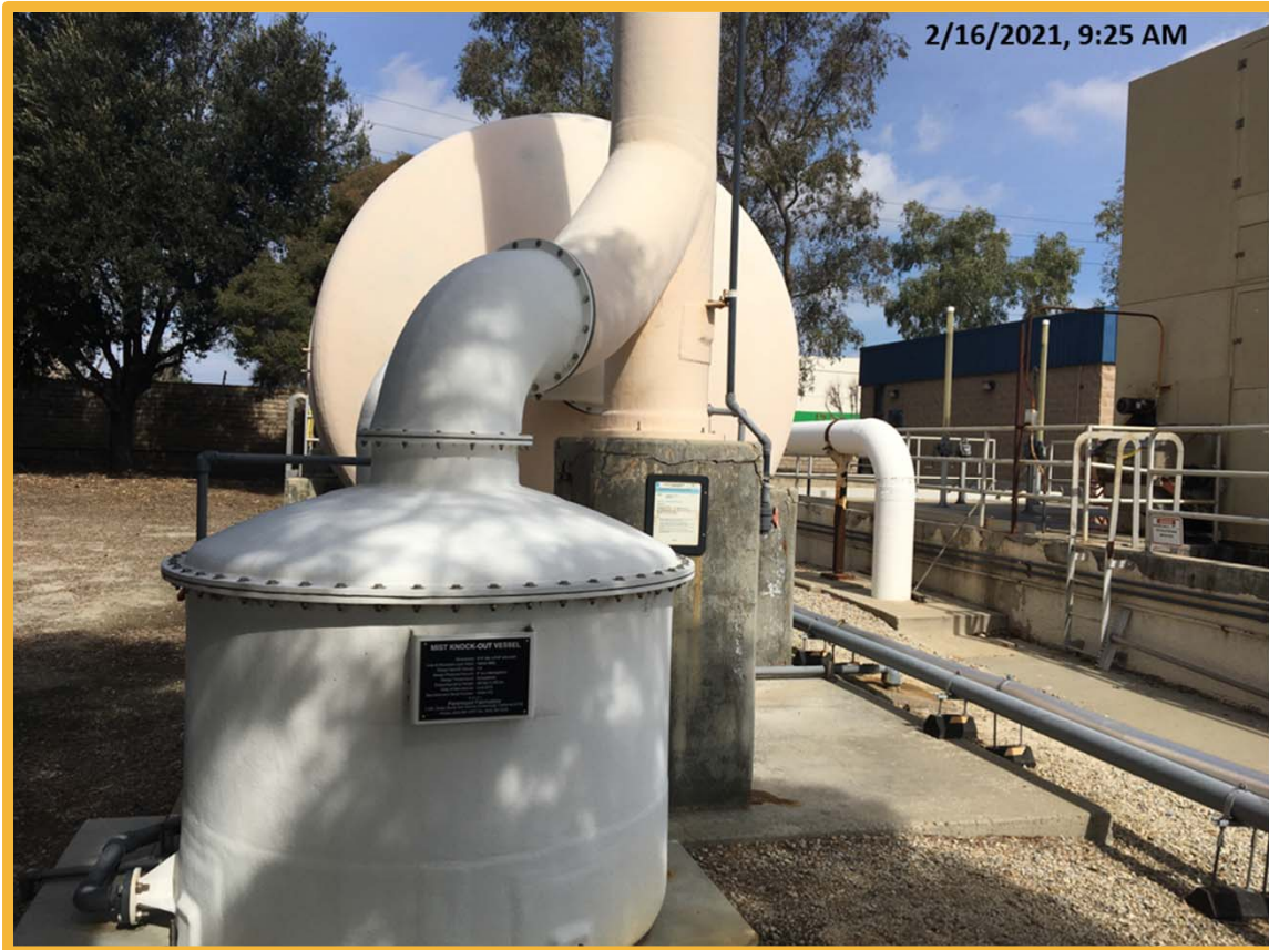
Horizontal Chemical Odor Scrubber
