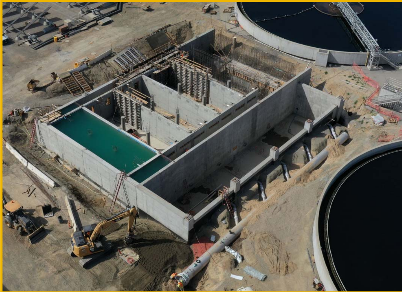
Membrane Bioreactor (MBR) Phase 1
