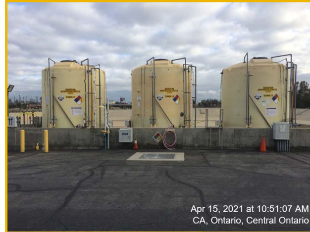
Existing Bleach Storage Tanks
