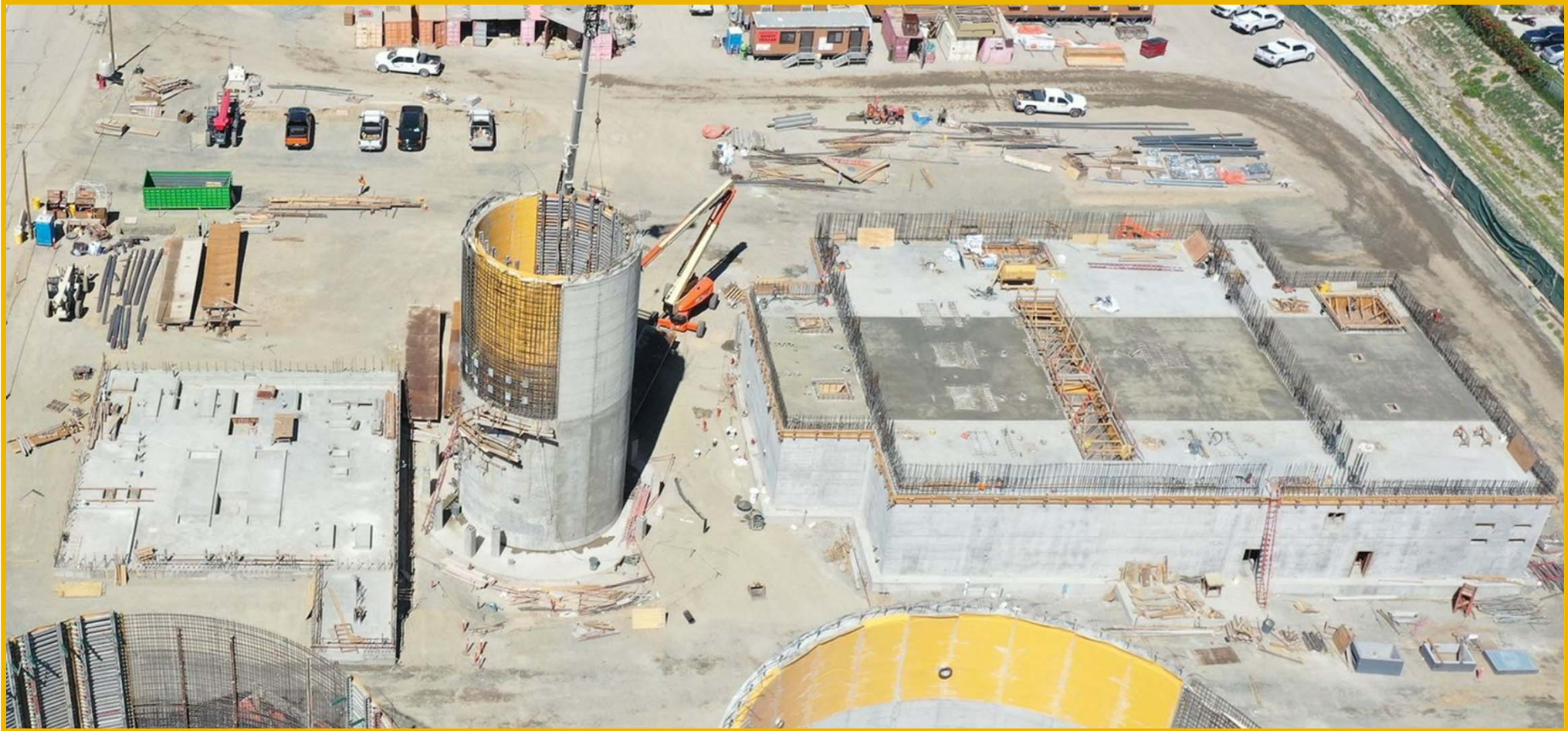
Acid Phase Digester
