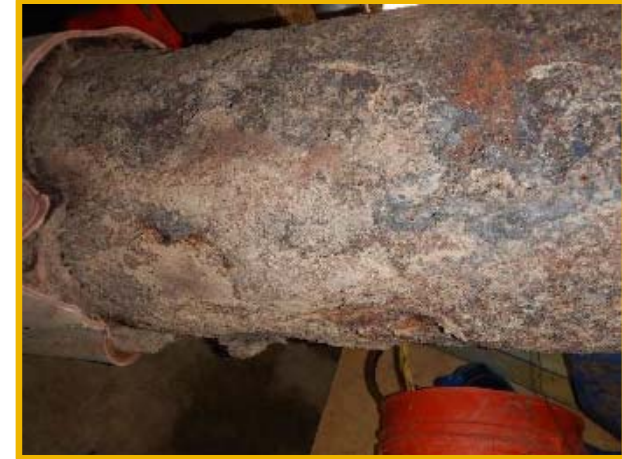
Corrosion on Pipeline
