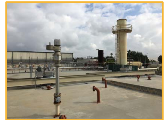
Solids Handling Facility Partial Views
