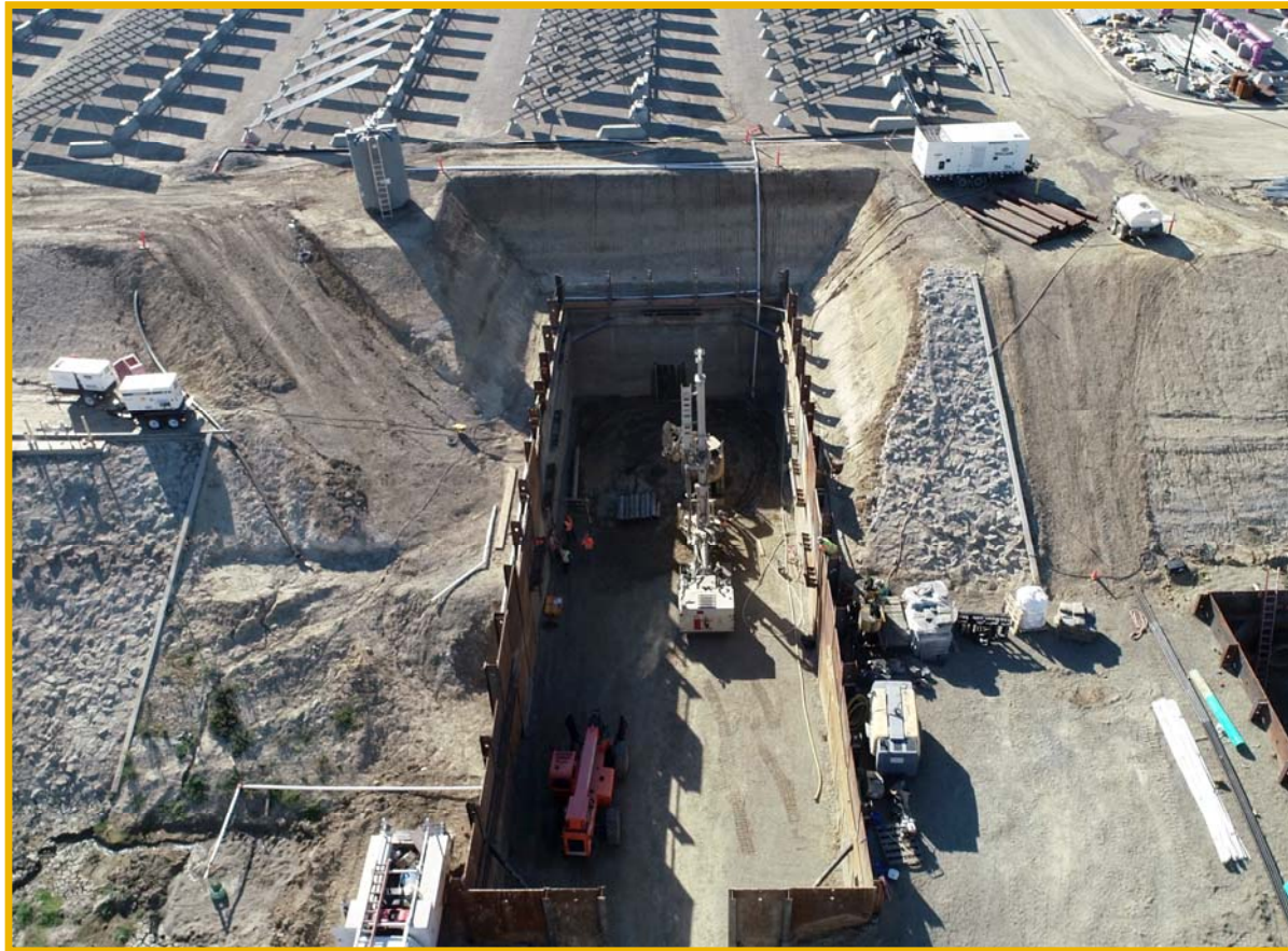
Emergency Overflow Pond Pump Station
