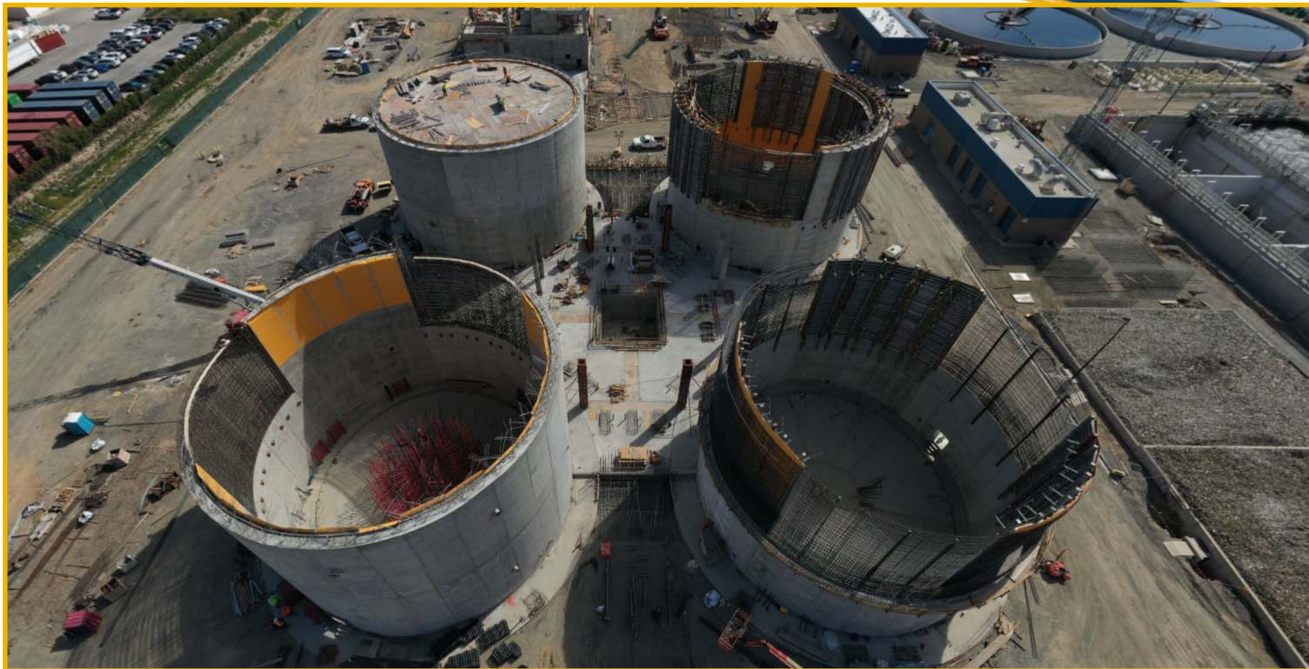
Gas Phase Digesters
