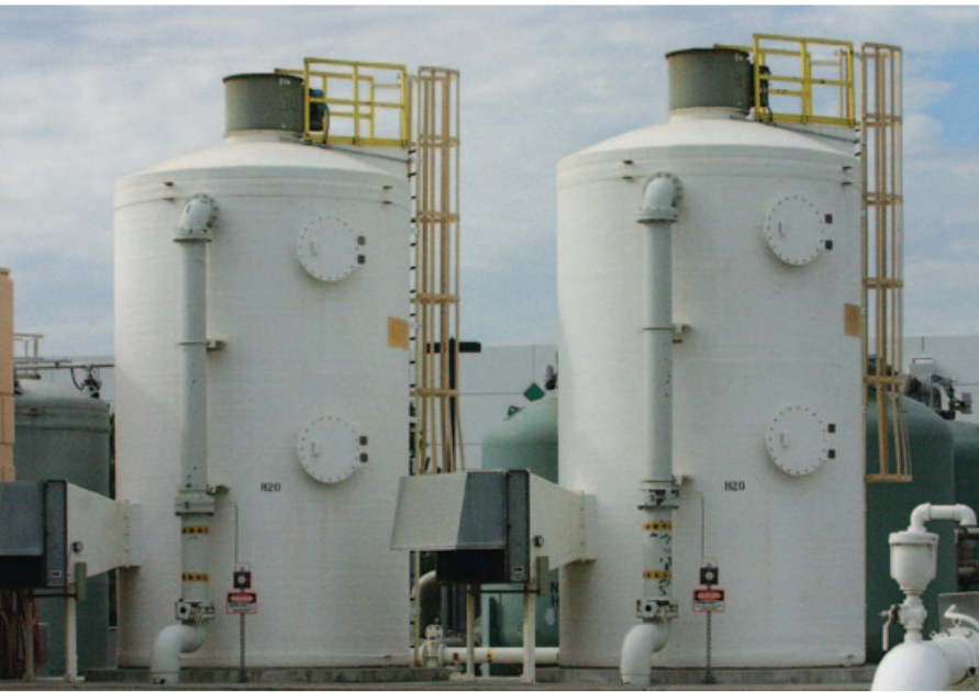
The Chino I Desalter began operation in 2001, and expanded production in 2005 from 8.4 to 14 million gallons a day.
