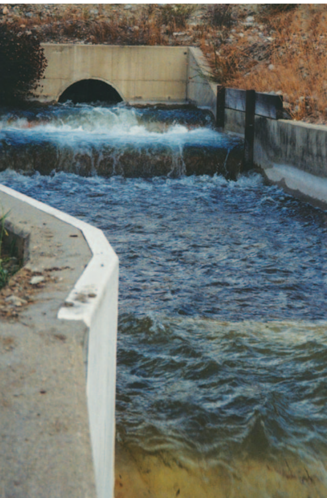
At Montclair 1, part of the Agency's groundwater recharge operations, water coming from San Antonio Channel flows over two stop log structures and a Parshall Flume which are used to measure cubic feet per second.
