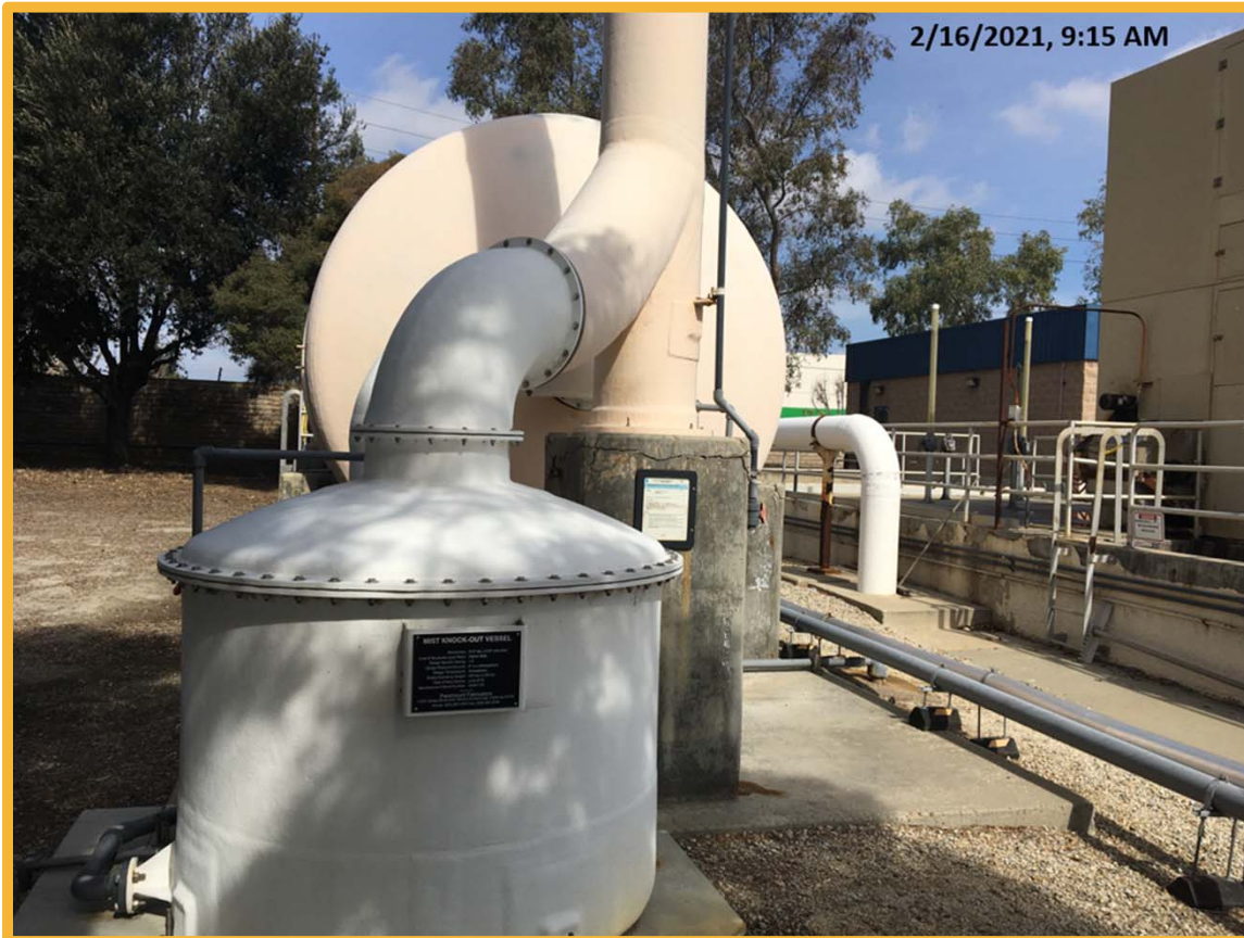
Chemical Odor Scrubber at Headworks
