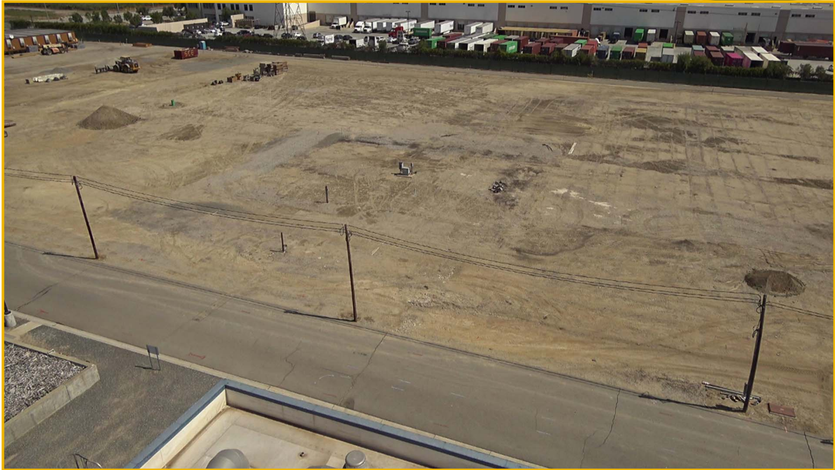
Digester Area Time-Lapse September 2020 - May 2021
