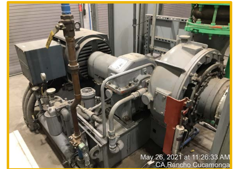
Existing Kawasaki Blower
