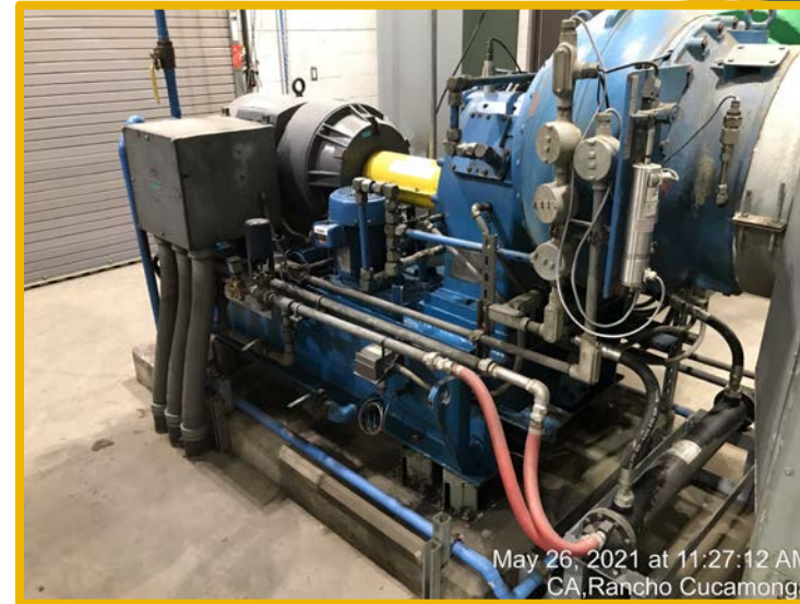
Existing Turblex Blower
