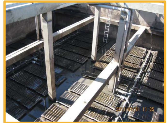
RP-1 Aeration Panel Diffusers
