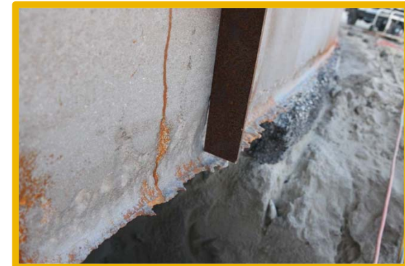
Visible Corrosion Damage on Bottom Plate Extension
