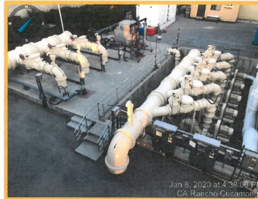
Influent Pump Station
