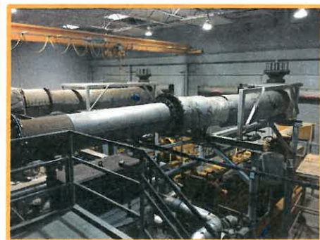
REEP Exhaust Piping
