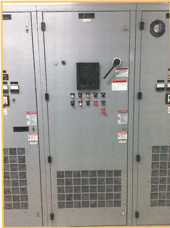
Influent Pump Control Center
