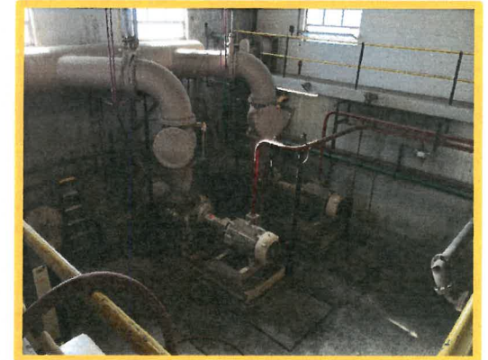
Obsolete pumps, equipment, and piping
