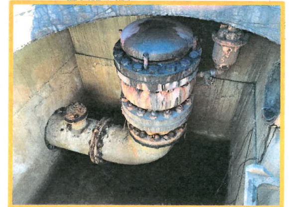
Existing Air Vac in Vault
