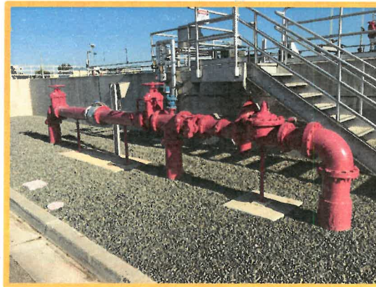
RP-5 Recycled Water Piping
