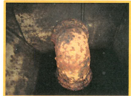
Corroded pipe in pump station wet well
