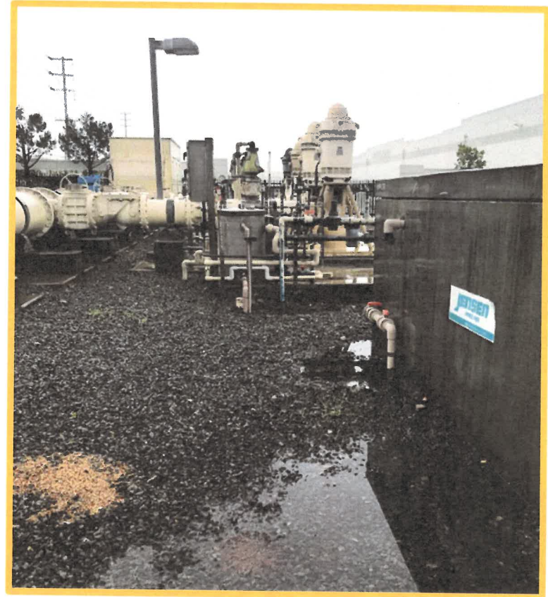
Lift Station Pumps
