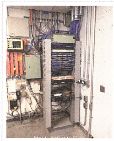
RP-4 SCADA Migration Project
