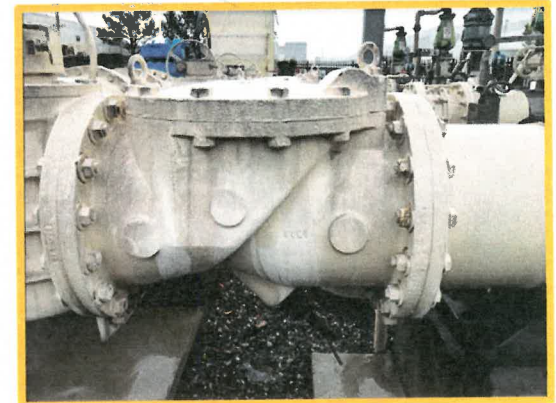
San Bernardino Lift Station Valve Connection
