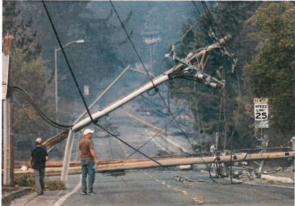
Power Lines Falling Onto Trees
