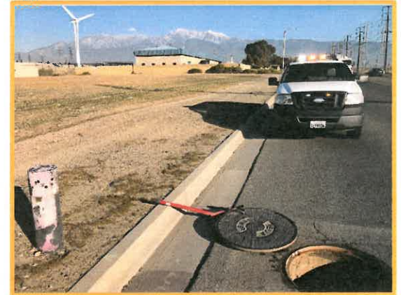
Air Relief Valve in Etiwanda Ave.
