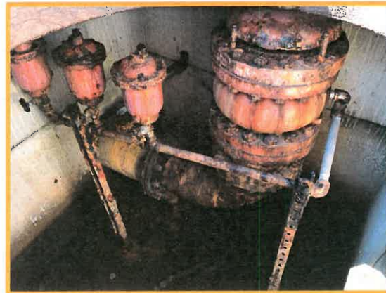
Air Relief Valves to be Replaced
