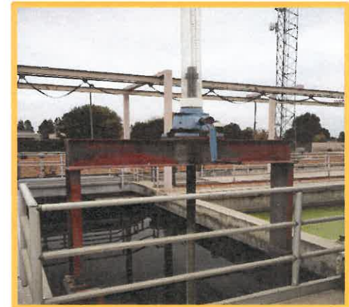
Corroded Isolation Gates at the Filters
