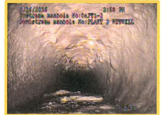
Buildup in 18" Effluent Pipeline
