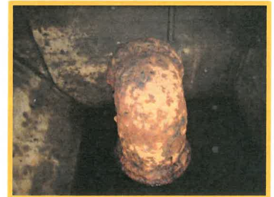
Corroded Pipe in Pump Station Wet Well
