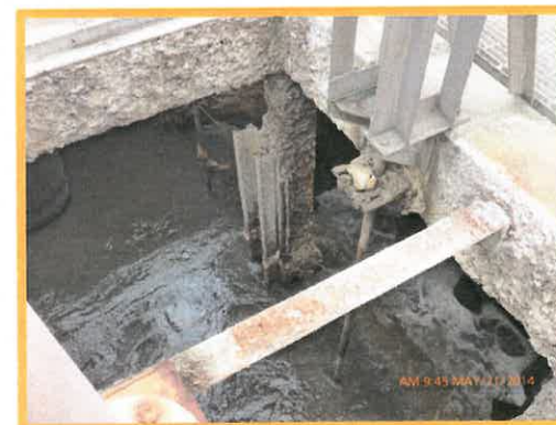
Exposed Rebar in Grating at Support Beam
