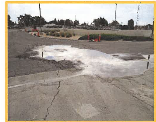
Surface Cracks and Drainage Issues
