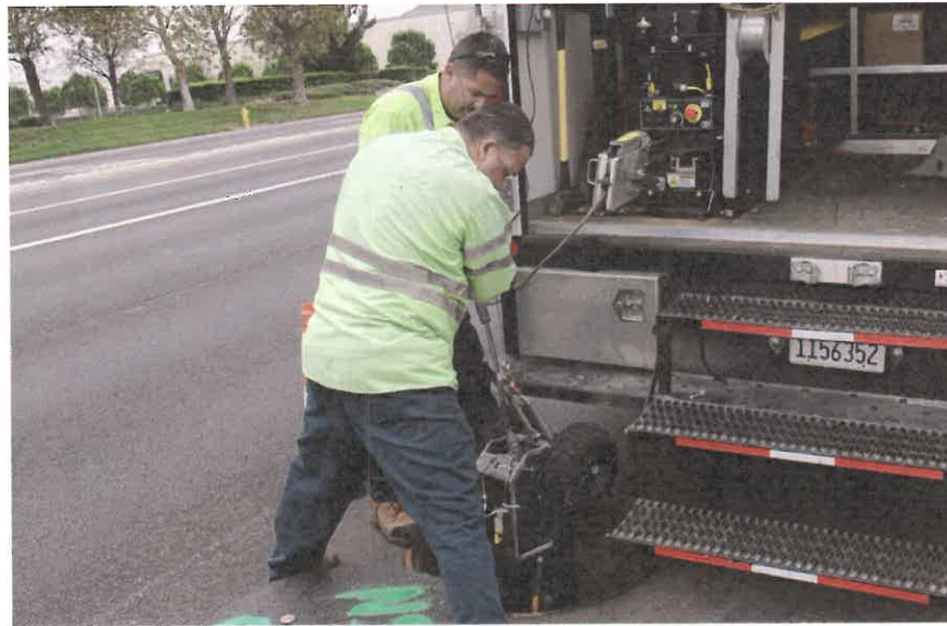
Sewer Collection Video
