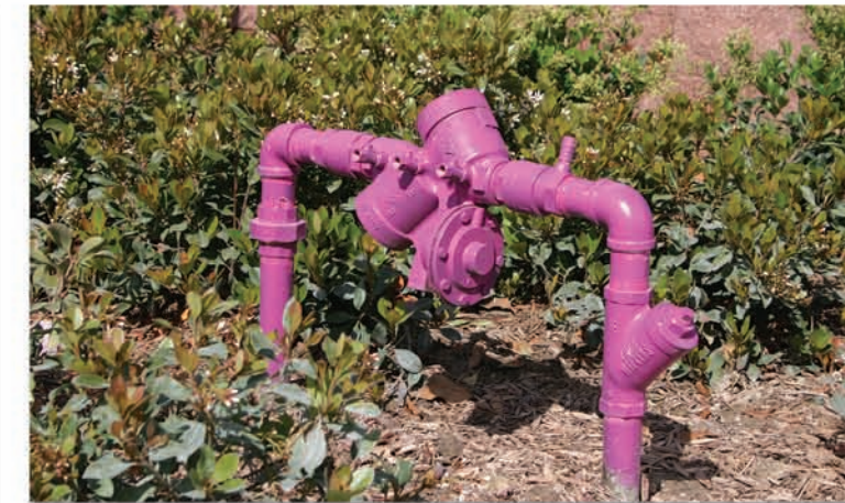
When you see a purple pipe, you see recycled water being used. Recycled water is 100% water conservation. It is helping drought-proof our region.
