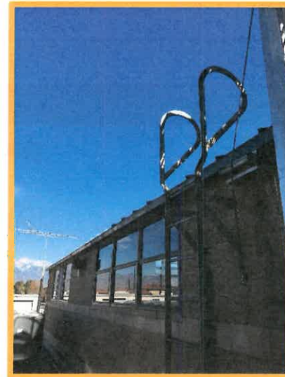
Access Ladder to HVAC Units
