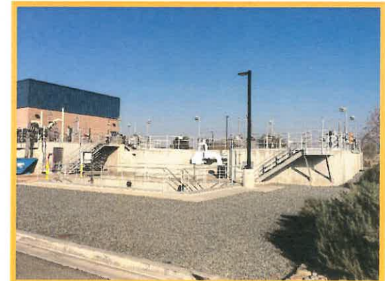
New Lights at RP-5 Headworks
