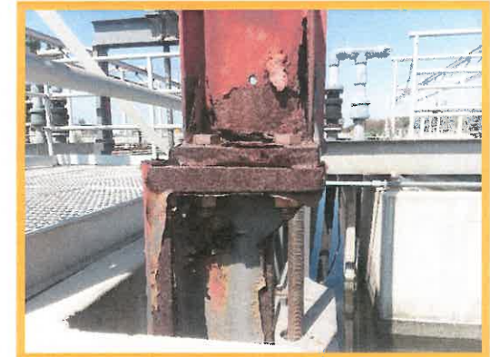
Corroded Gates at the Filters
