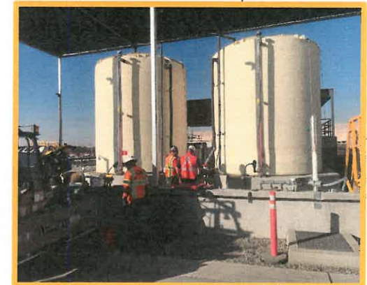
New Chemical Storage Tanks
