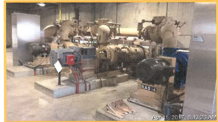
RAS Pump Station for Secondary Treatment System
