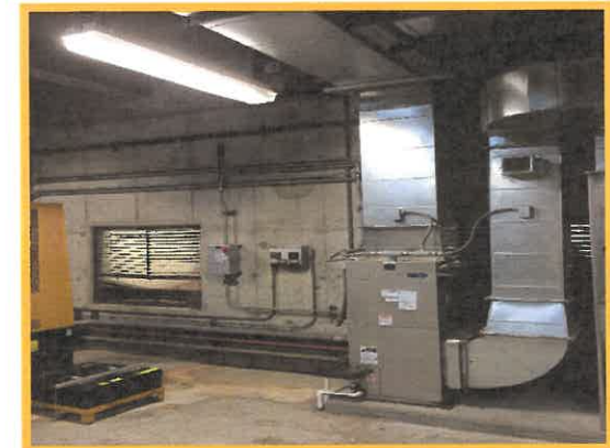
Existing HVAC Ducting to be Modified
