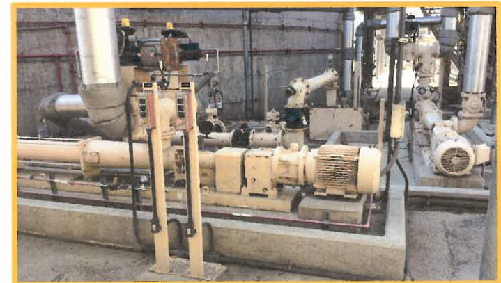
Sludge Transfer Pump at Digester Area
