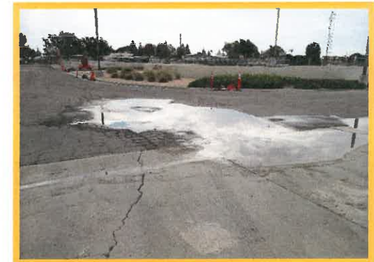
Cracked Pavement and Ponding
