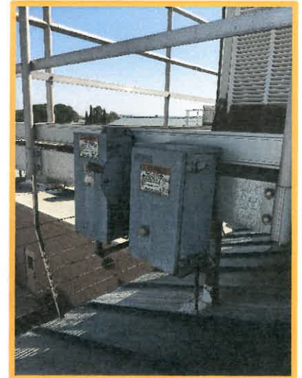
Disconnect and Motor Control Panels
