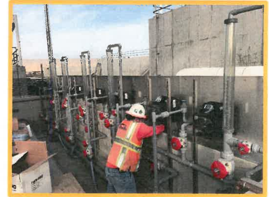
New Chemical Pumps
