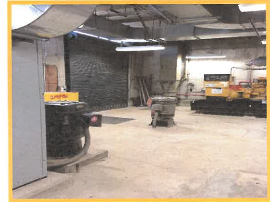
Existing Pump No. 3
