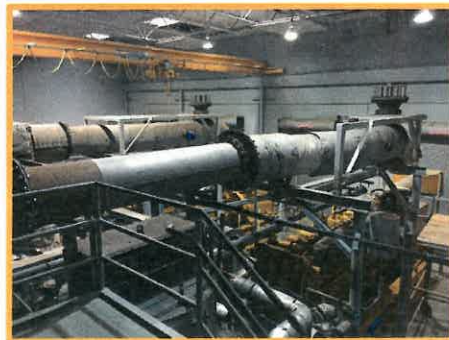
REEP Exhaust Piping
