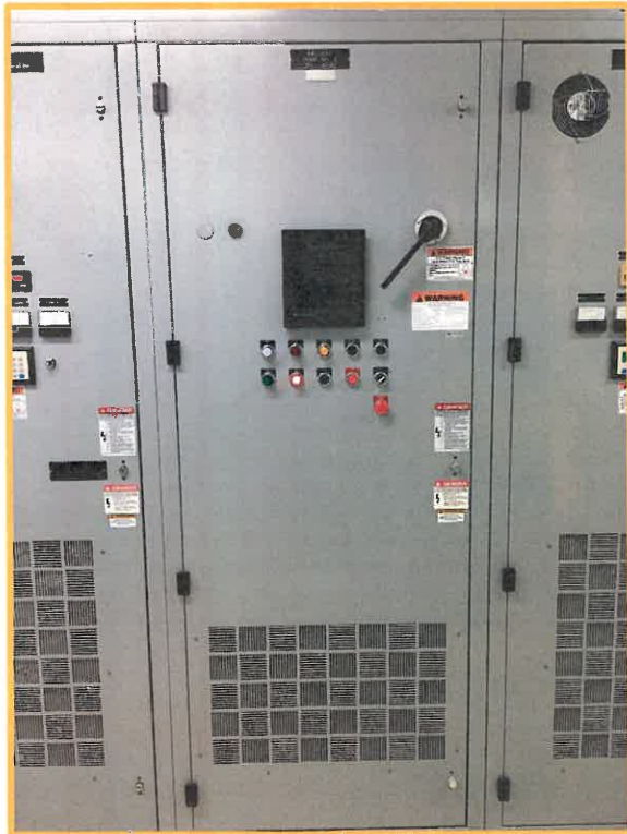
Influent Pump Control Center
