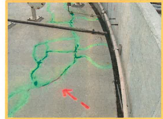
Digester No. 6 Partial Roof Cracks
