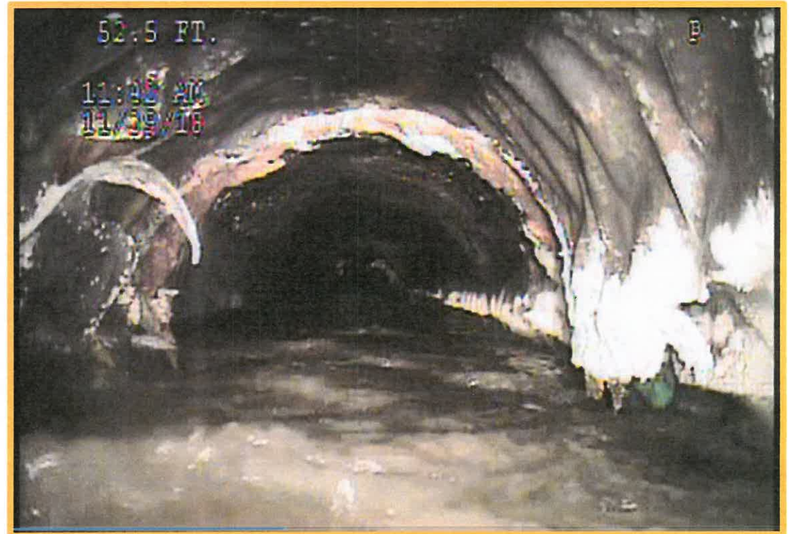
Pipeline Lining Deterioration
