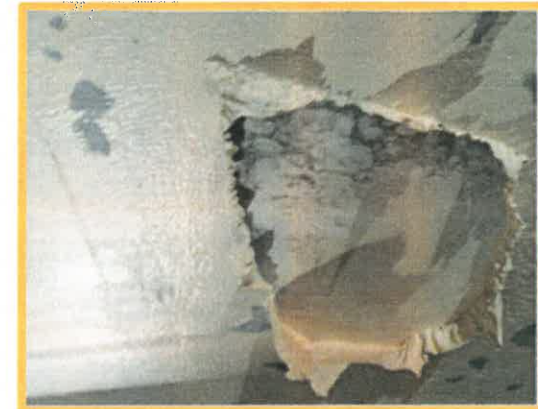
Failed Internal Roof Coating
