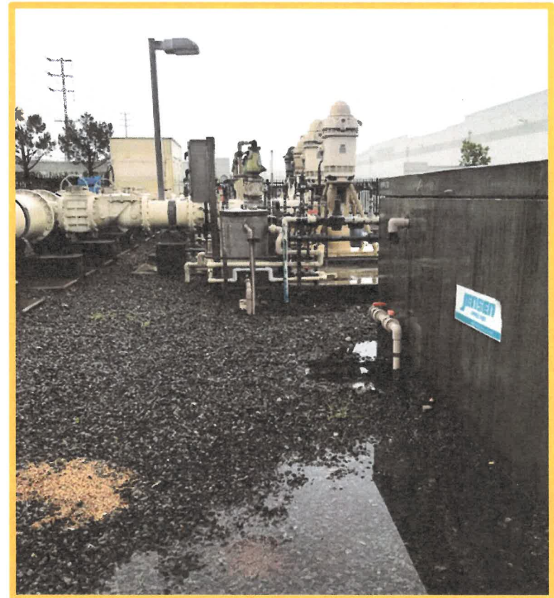
Lift Station Pumps
