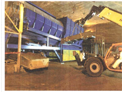
IERCF Compost Screening Replacement Trommel Screen Video
