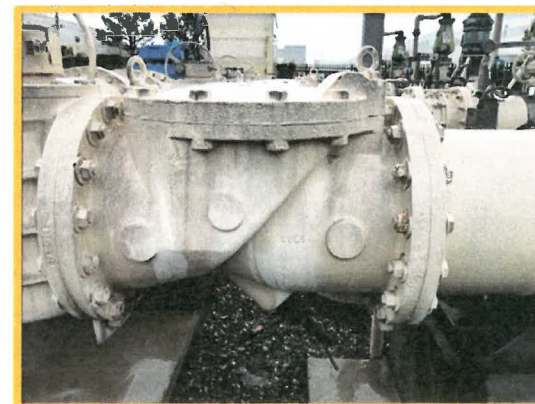
San Bernardino Lift Station Valve Connection
