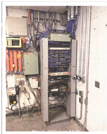
RP-4 SCADA Migration Project
