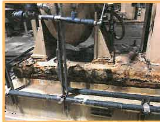
Corroded Sludge Pump Base
