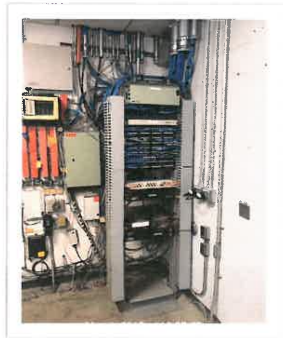
RP-4 SCADA Migration Project
