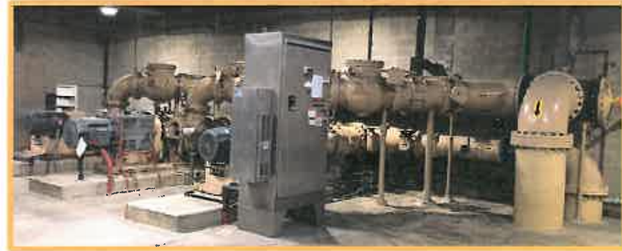
Sludge Pump Equipment and Appurtenances
