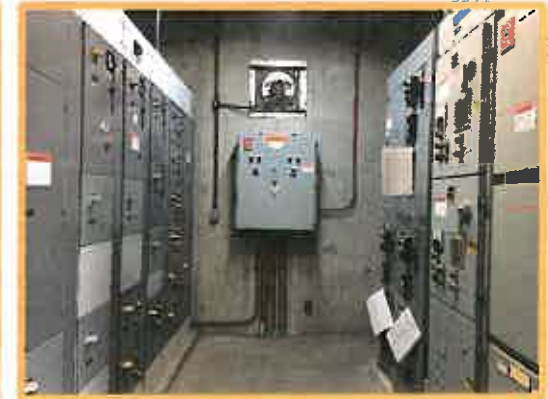
Outdated Motor Control Center
