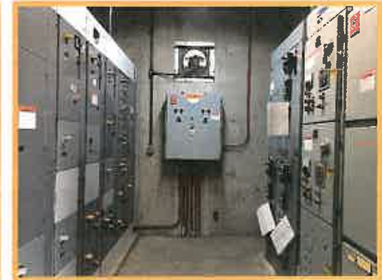
Outdated Motor Control Center
