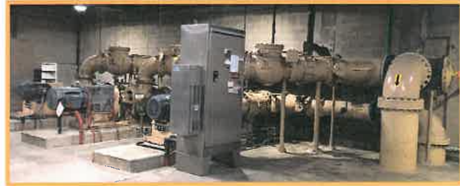
Sludge Pump Equipment and Appurtenances
