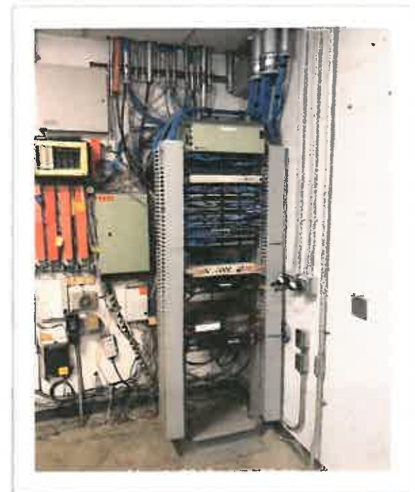
RP-4 SCADA Migration Project
