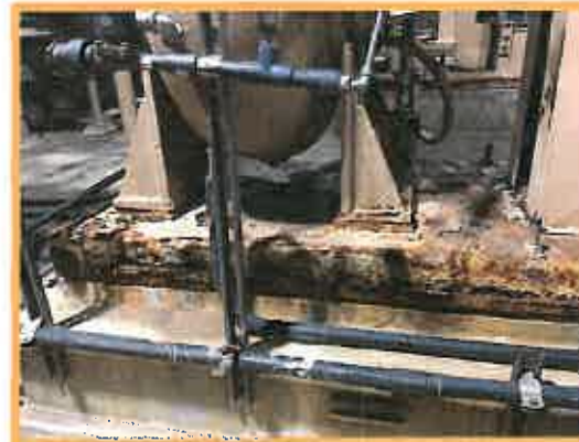
Corroded Sludge Pump Base
