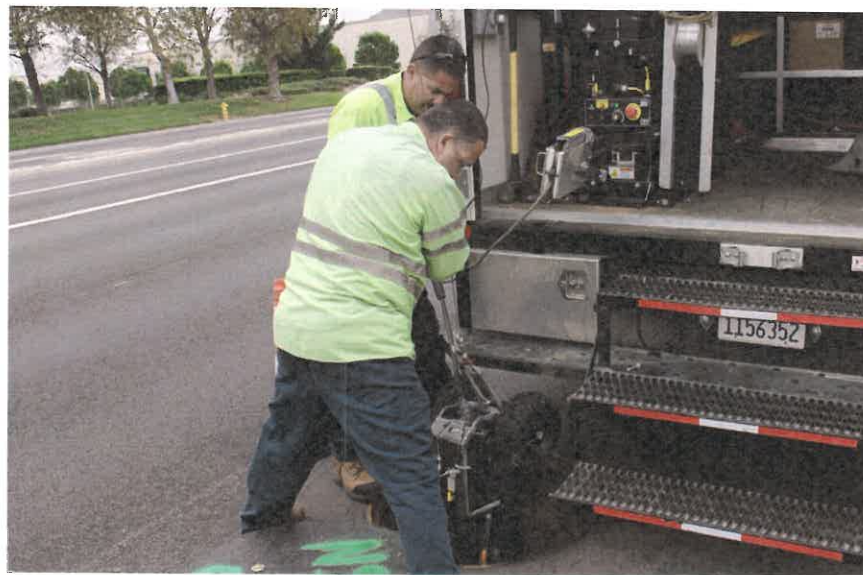
Sewer Collection Video
