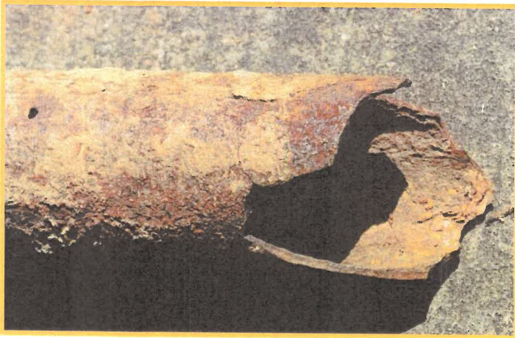
Example of Extremely Corroded Pipe
