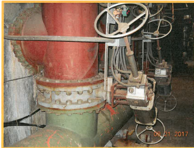
20-Inch Valve and Calcium Deposits
