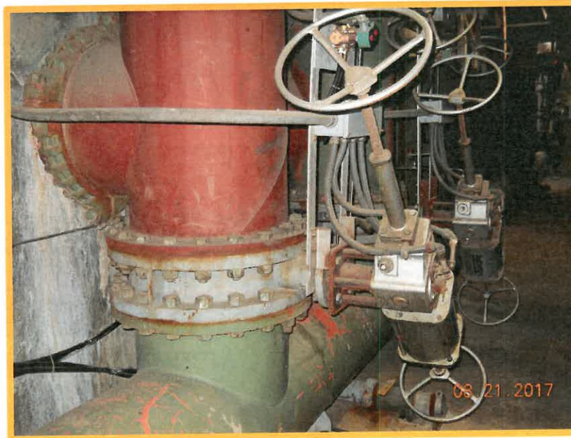
20-Inch Valve and Calcium Deposits
