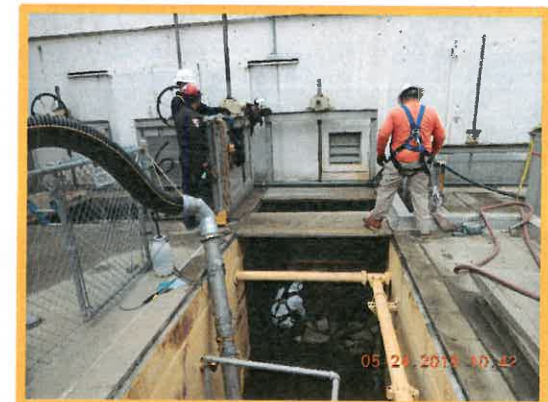
Contractor attempting to manage Leakage
