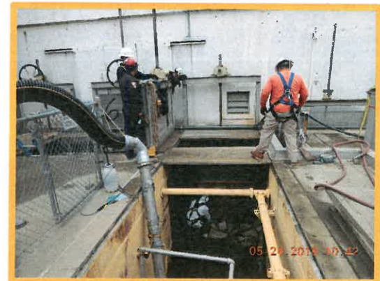
Contractor attempting to manage Leakage
