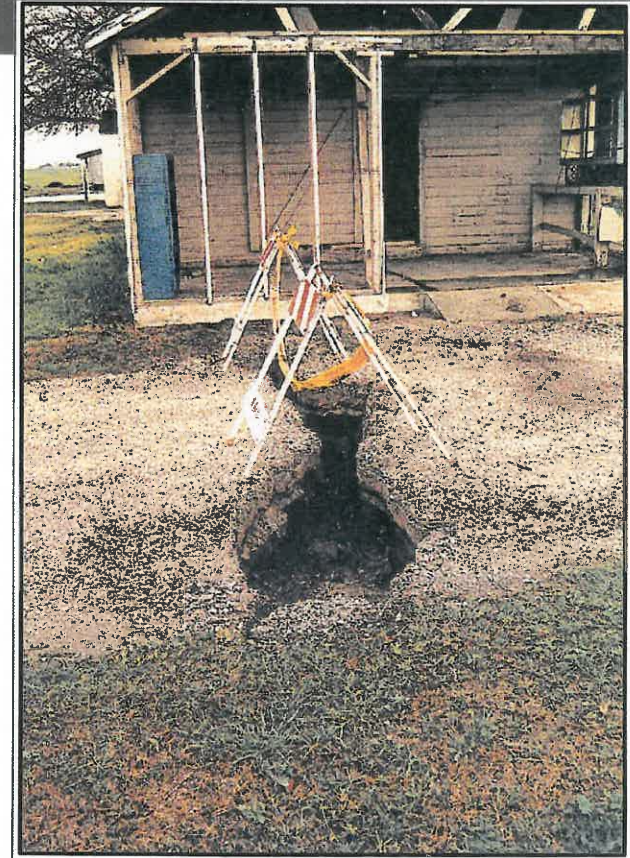
View of a fissure that developed beneath CIM facility in December 1992
