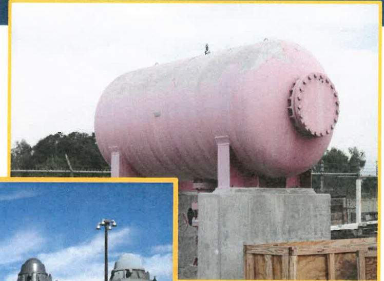
Existing 2,500 Gallon Surge Tank
