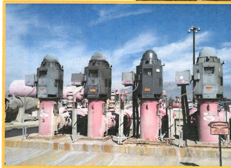
RP-1 Recycled Water Pump Station
