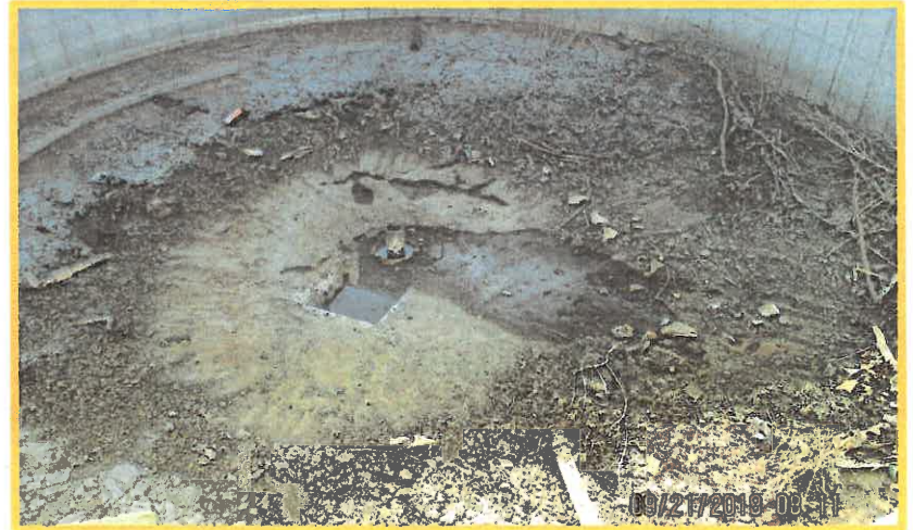
Ground Water Infiltration 09/21/18 8:11 AM
