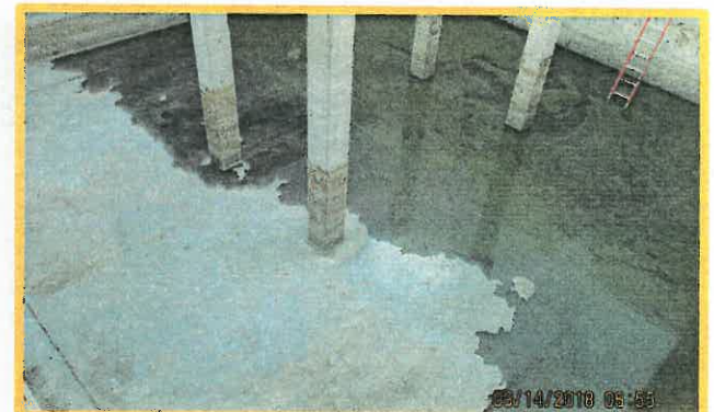
Ground Water Infiltration 09/14/18 6:55 AM
