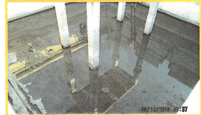
Ground Water Infiltration 09/13/18 7:37 AM
