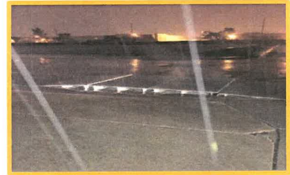
Vault Covers Floated During Winter 2017 Rain Event
