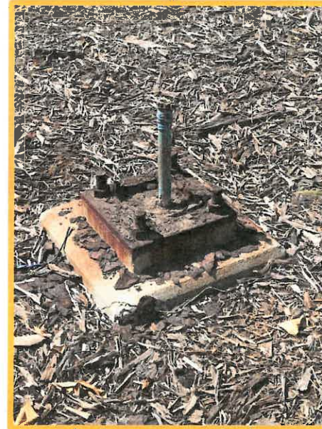
Existing Damaged Base
