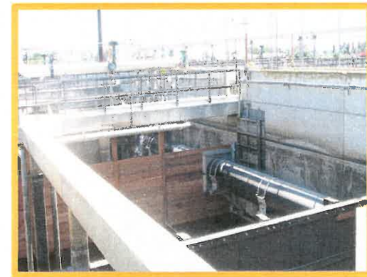
Baffle Walls and Mixed Liquor Return Pumps
