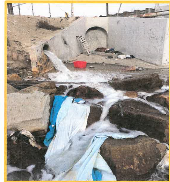
Existing Recycled Water Discharge
