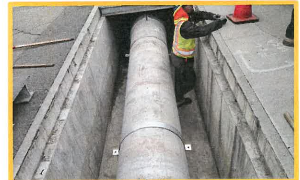
Straps Installed to Limit Duct's Displacement
