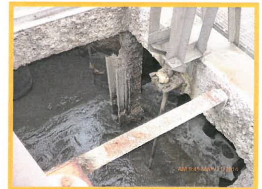
Distressed Diversion Structure
