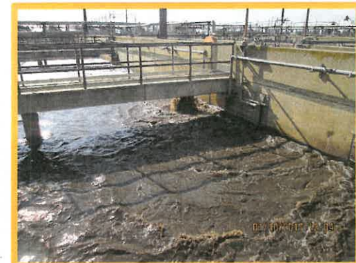
Mixed Liquor Return Pump Operating
