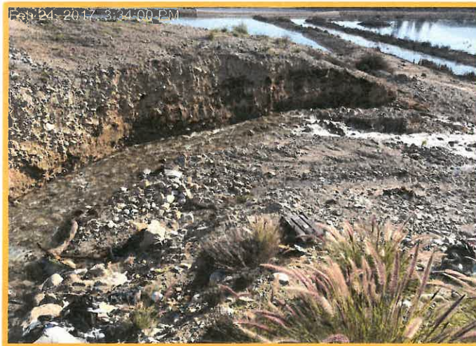
Existing Erosion in Unlined Channel
