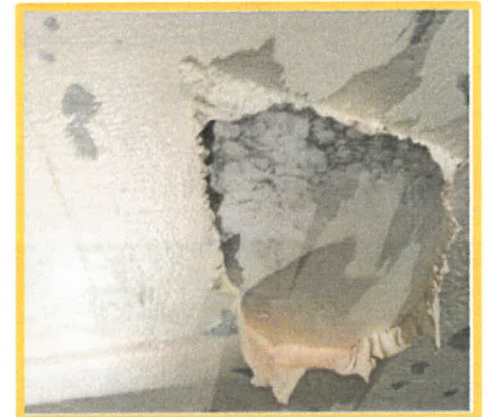
Failed Internal Roof Coating
