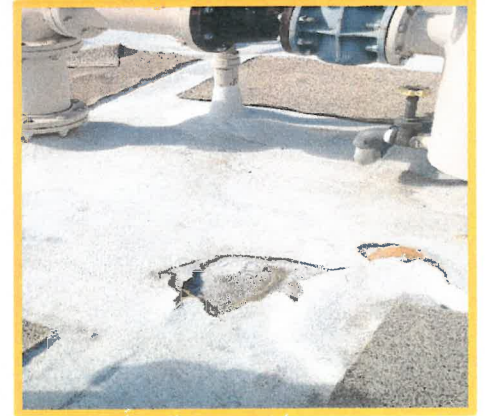
Cracking of Foam Roofing Insulation
