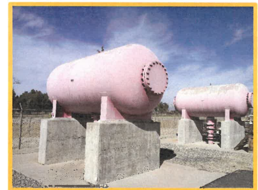
RP-1 Recycled Water Surge Tanks
