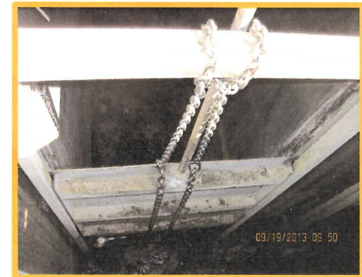
Gate Upstream of Headworks: Failed to Open
