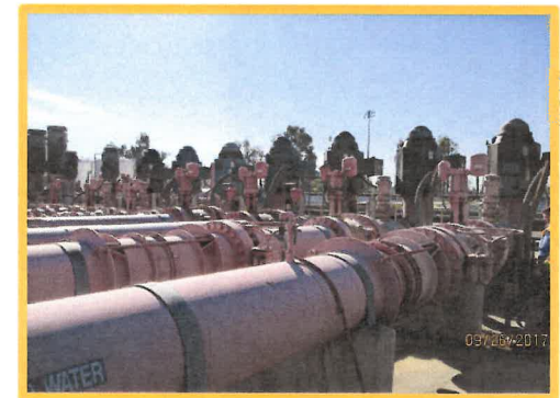
RP-1 Recycled Water Pumps
