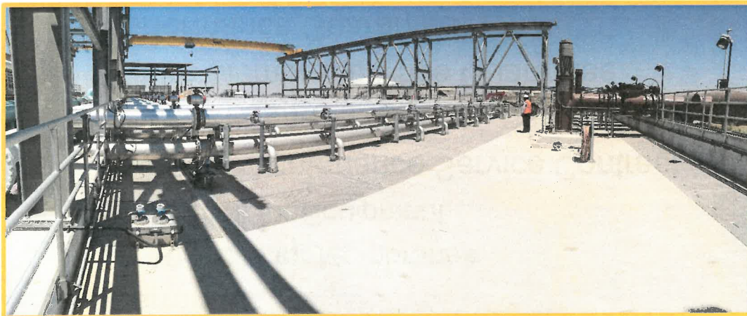
Visalia Water Recycling Facility Membrane Bio-Reactor System
