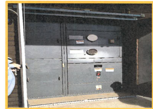
Outdated 480V Switchboard Board will be Replaced
