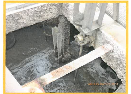
Distressed Diversion Structure
