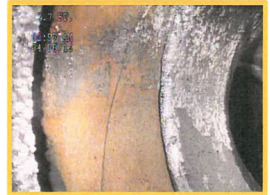
Minor Fracture within the 36" Piping
