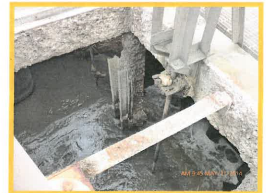
Distressed Diversion Structure
