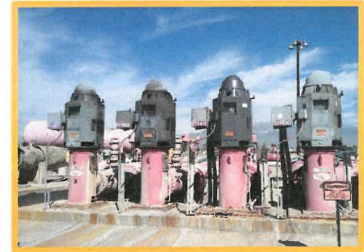
RP-1 1158 RWPS 400 HP Pumps
