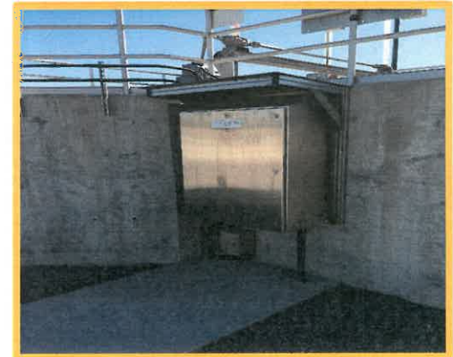
New Control Panel
