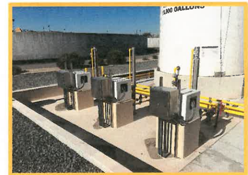
New Chemical Pumps
