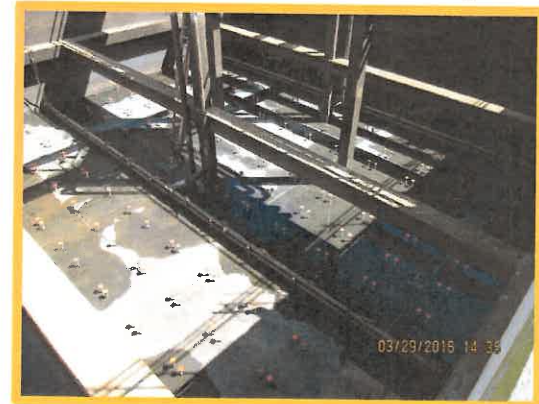
PVC air header piping
