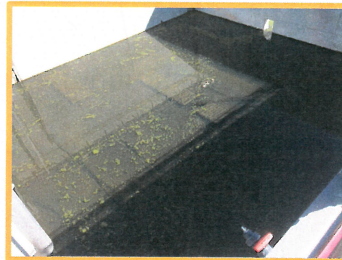
RP-5 Aeration Basin with Failed Diffusers
