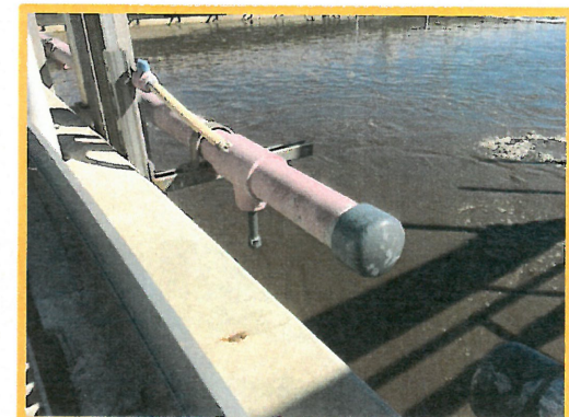
Out of Service Surface Sprayer Pipeline
