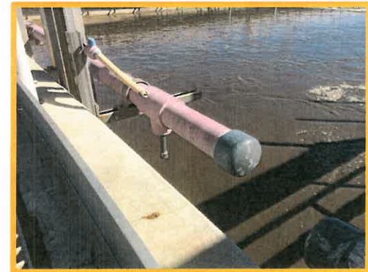
Out of Service Surface Sprayer Pipeline
