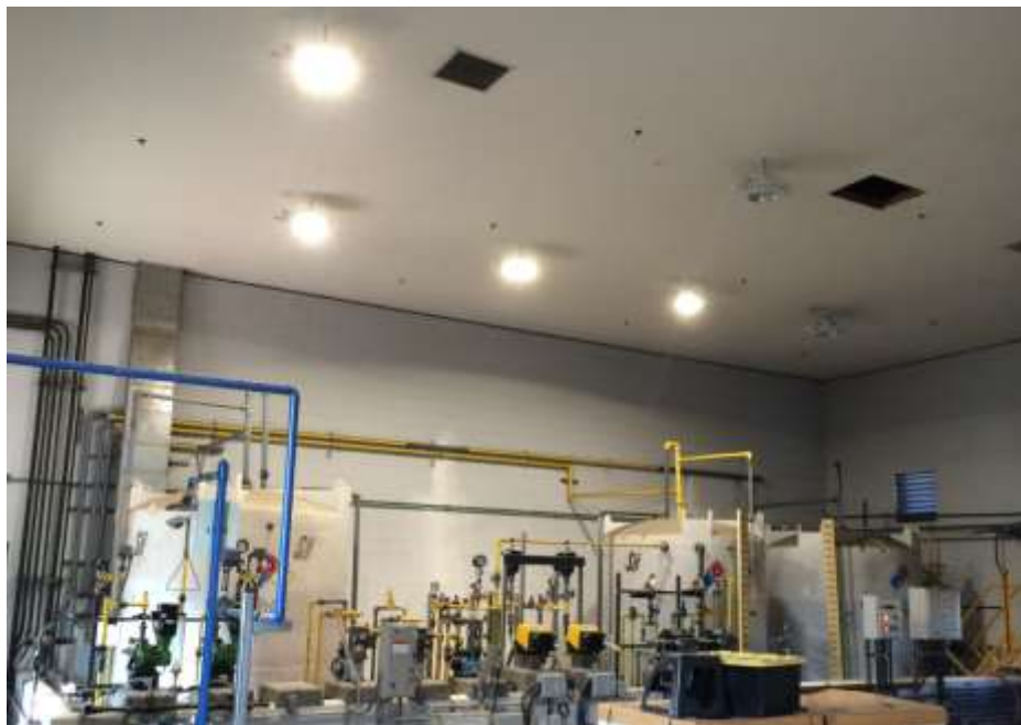
LEDs installed at RP4's chemical storage room
