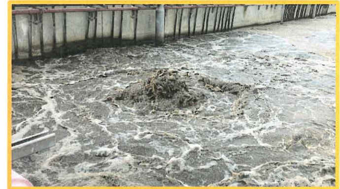
Aeration Basin Surface Boil
