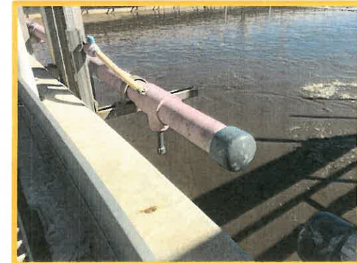
Out of Service Surface Sprayer Pipeline
