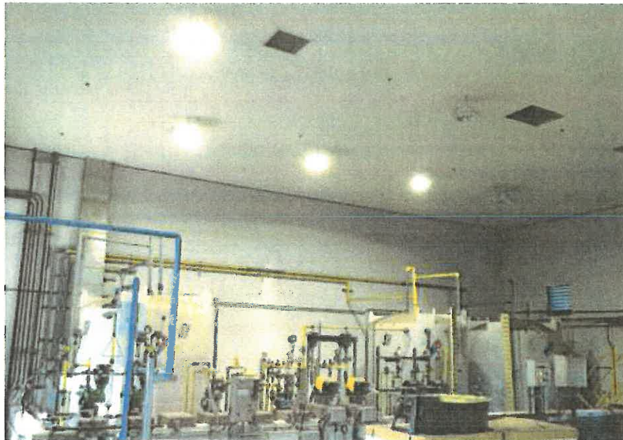
LEDs installed at RP4's chemical storage room
