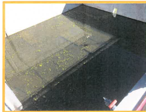
RP-5 Aeration Basin with Failed Diffusers
