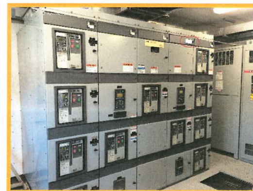
Front of Switchgear
