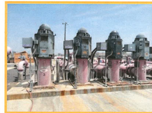
Recycled Water Pump Station Motors
