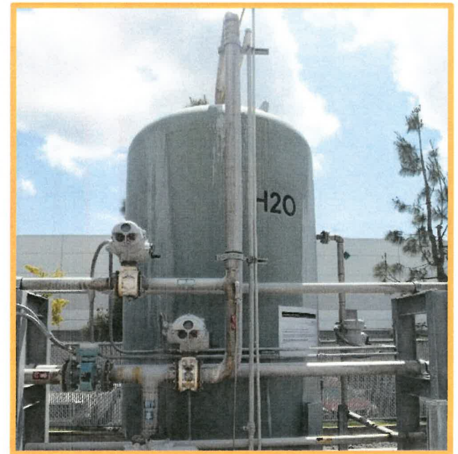
Deterioration of Surface Coating on Process Vessel
