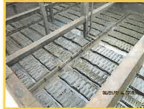
Drained Aeration Train No. 2
