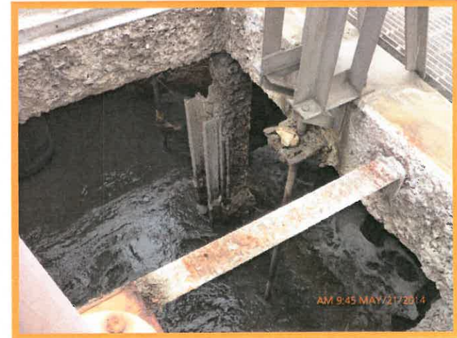
Exposed Rebar In Grating At Support Beam
