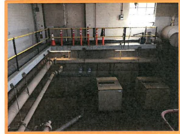
Plant No. 2 Basement Piping
