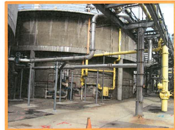
Bottleneck at Digester Area
