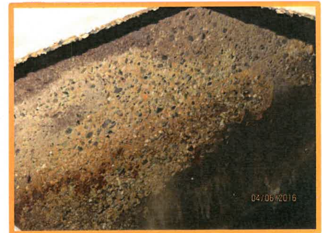
IPS Wet Well Concrete Corrosion
