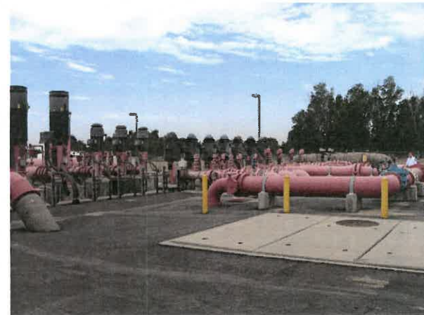
RP-1 Recycled Water Pump Station
