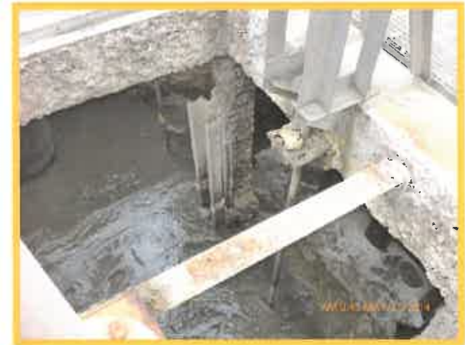
EXPOSED REBAR IN GRATING AT SUPPORT BEAM
