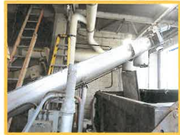
GRIT PROCESSING EQUIPMENT
