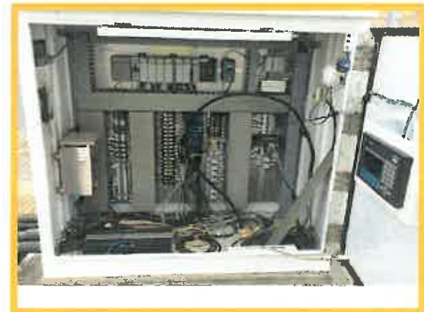
TURNER BASIN CONTROL PANEL
