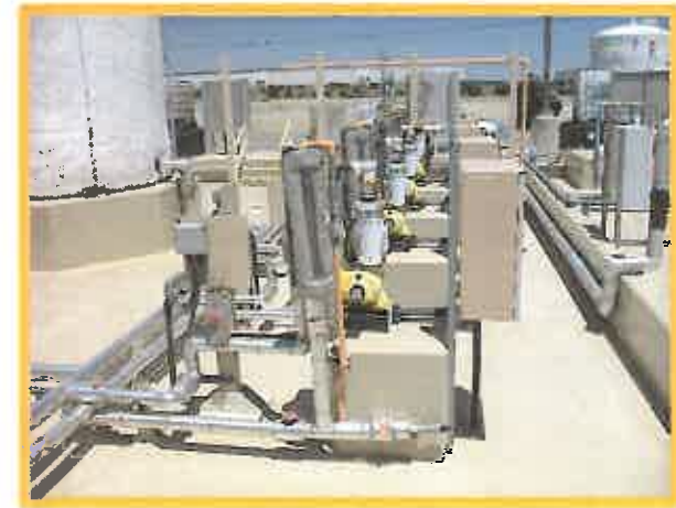
EXISTING SHS PUMPS TO BE REPLACED
