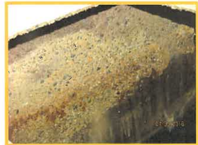
IPS WET WELL CONCRETE CORROSION
