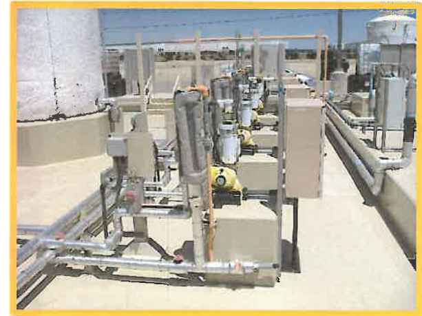
EXISTING SHS PUMPS TO BE REPLACED
