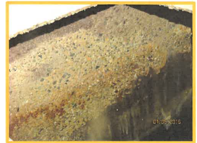
IPS WET WELL CONCRETE CORROSION
