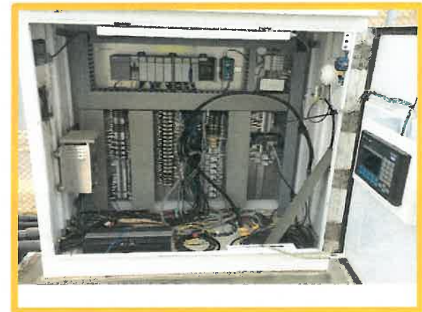
TURNER BASIN CONTROL PANEL
