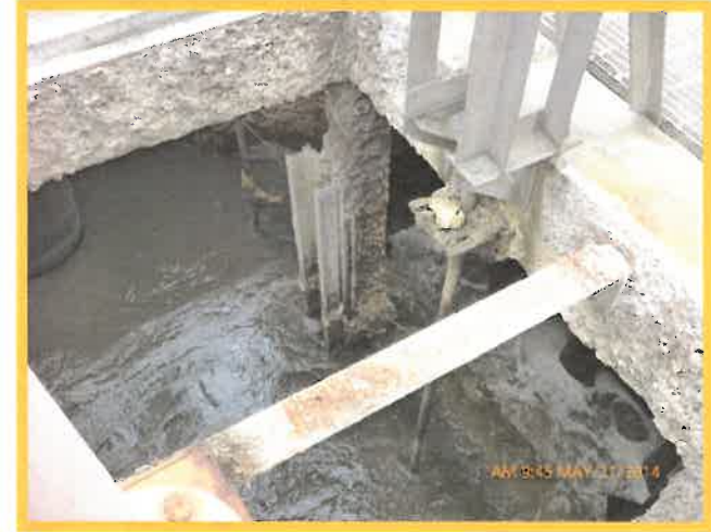
EXPOSED REBAR IN GRATING AT SUPPORT BEAM
