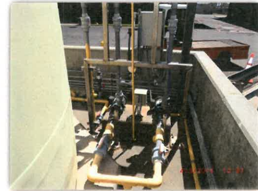
Bleach Loop Pumps
