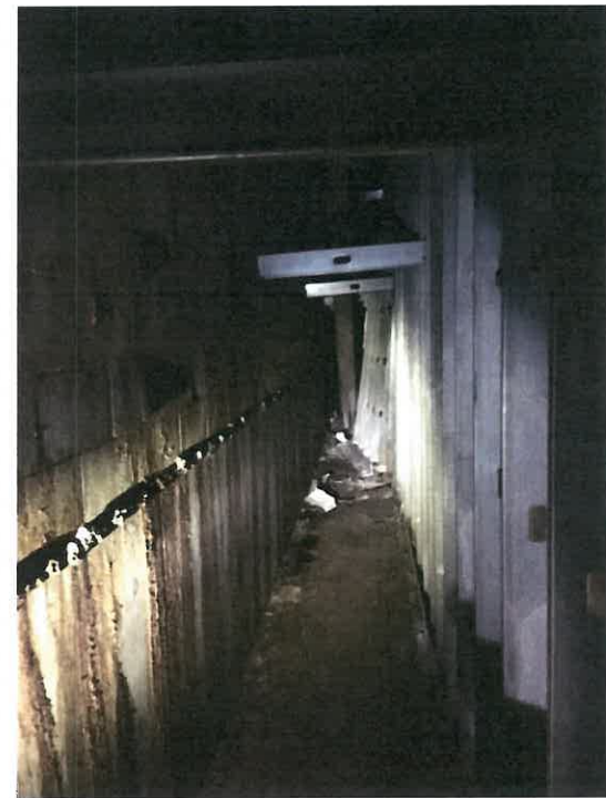
Air Duct Failure: Contractor secured and sealed the duct wall
