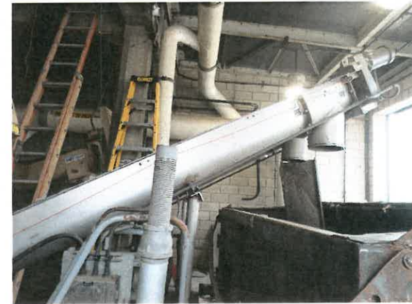
Grit Processing Equipment
