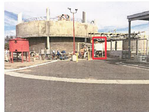
Acid Phase Digester Iron Sponge
