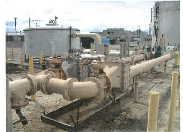
Digester Gas Piping to the Flare
