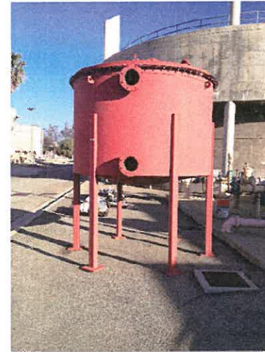
Acid Phase Digester Iron Sponge
