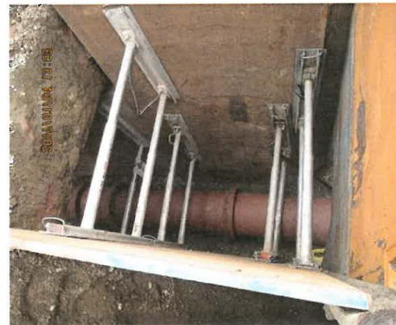
18-in Pipeline Between Manholes
