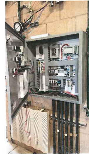
Control Panel at 1630 West
