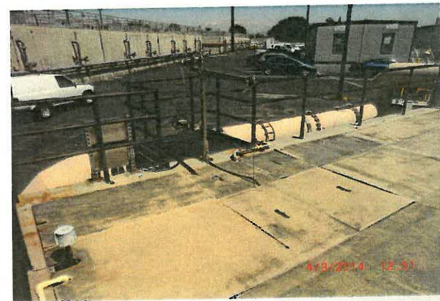
Existing NES dosing location
