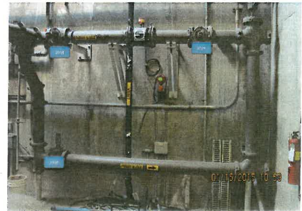
Primary Sludge Pipes
