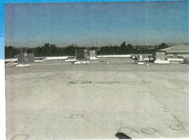
Existing Deteriorated TPO Roof Membrane
