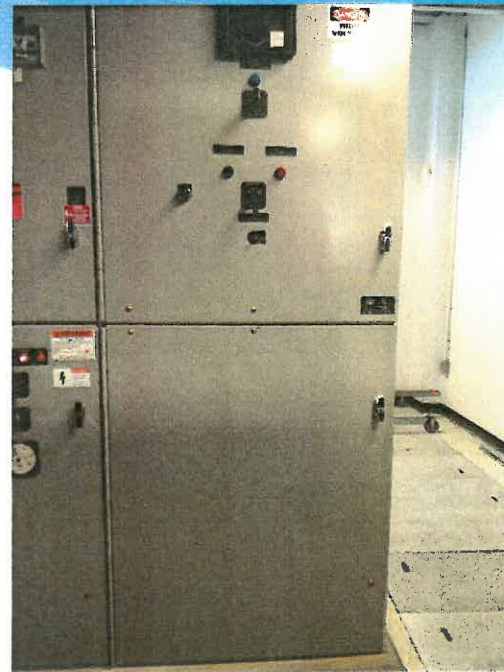
Vertical Switchgear Inside the Power Reliability Building
