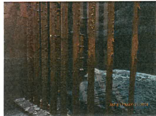
Intermediate PS Wet Well Coating Failure on Steel Bar Screen
