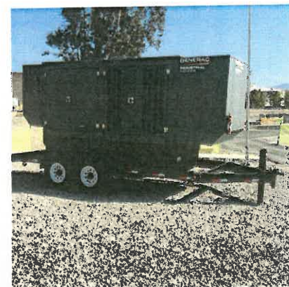
Existing Portable Generator
