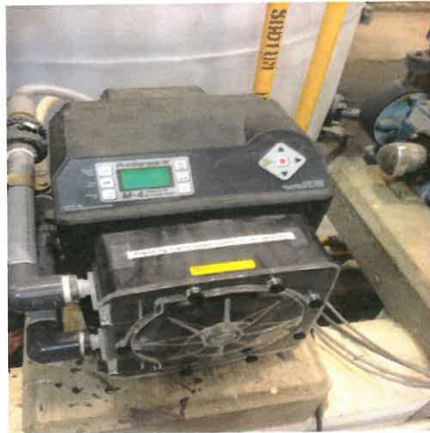
Existing Diaphragm Pump
