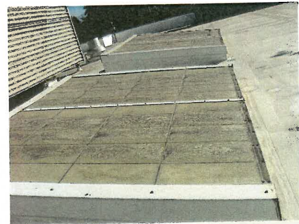
Discolored and Delaminating Skylight
