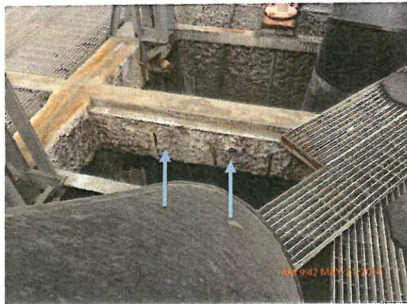
Exposed Rebar in Grating in Support Beam
