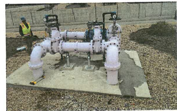
Completed RP-1 Utility Water Flow Meter
