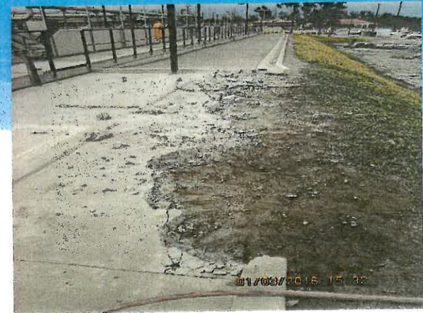
Power Center Pad
