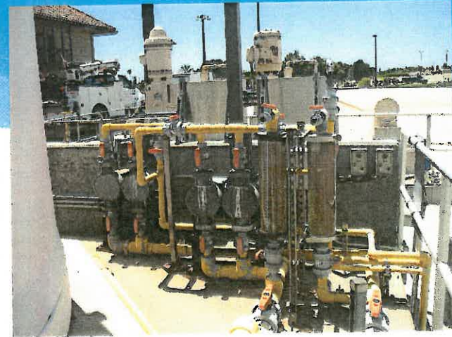
Existing TP-1 FM-1 Bleach Pumps
