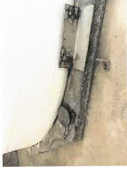
Damaged Concrete Pad Under Tank
