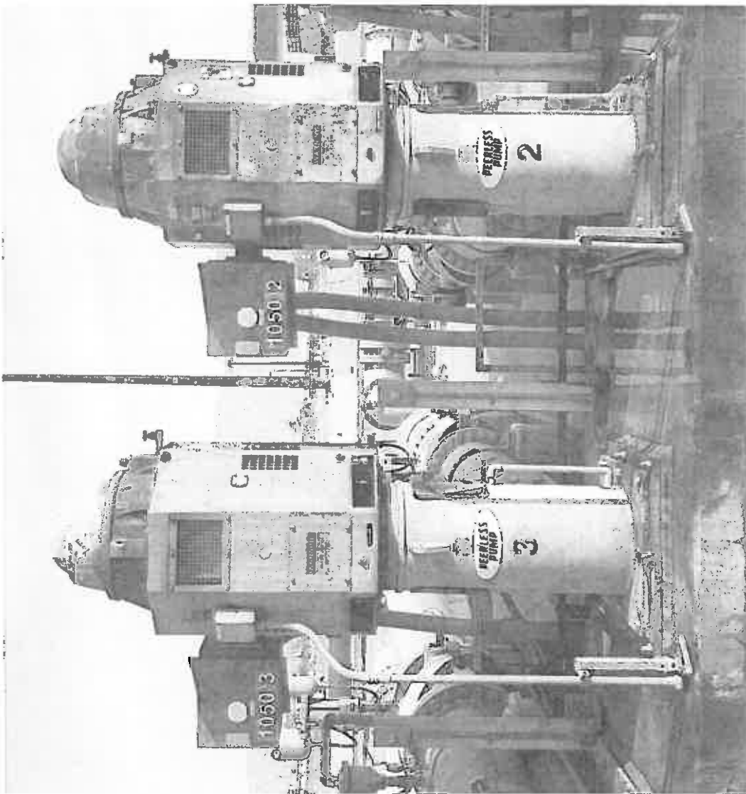
RP-1 1050 Pressure Zone Pumps No. 2 & 3
