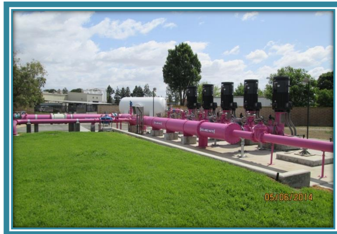
CARBON CANYON WATER RECLAMATION FACILITY – RECYCLED WATER PUMP STATION
