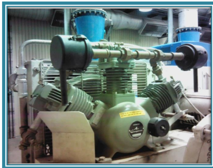
REGIONAL WATER RECYCLING FACILITY NO. 1 – AERATION BASIN COMPRESSOR
