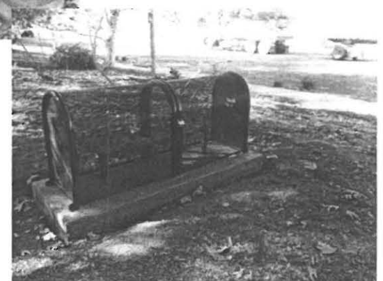
HQ-B Backflow Device - After
